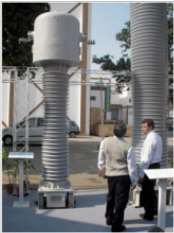
High-tech, 550kV, SF6 gas insulated, instrument transformer technology tie-up facilitated by Ace.
